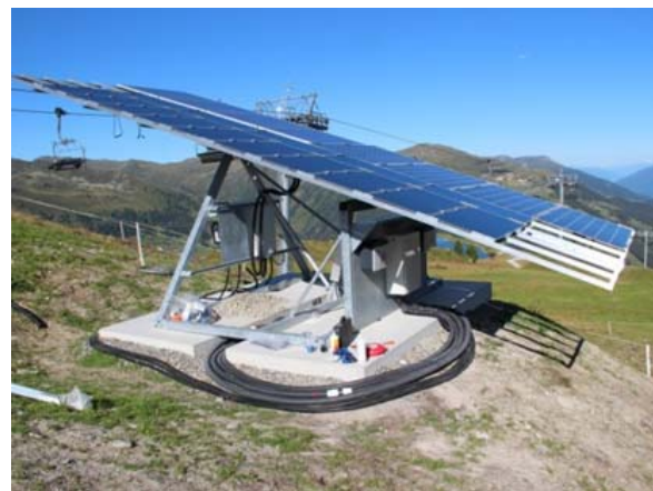
Fig. 2: High alpine Photovoltaic system (© alpS GmbH)
