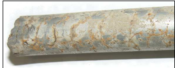
Fig. 2: Corroded heat exchanger tube (copyright: BIOENERGY 2020+)
