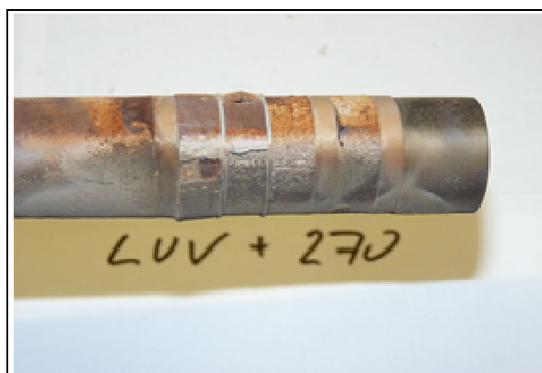
Fig. 1: Online corrosion probe after application in biomass heating plant (copyright: BIOENERGY 2020+)
