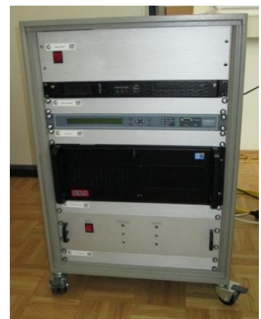
Figure 2: Indoor-unit of the Alphasat Ground Propagation Terminal
